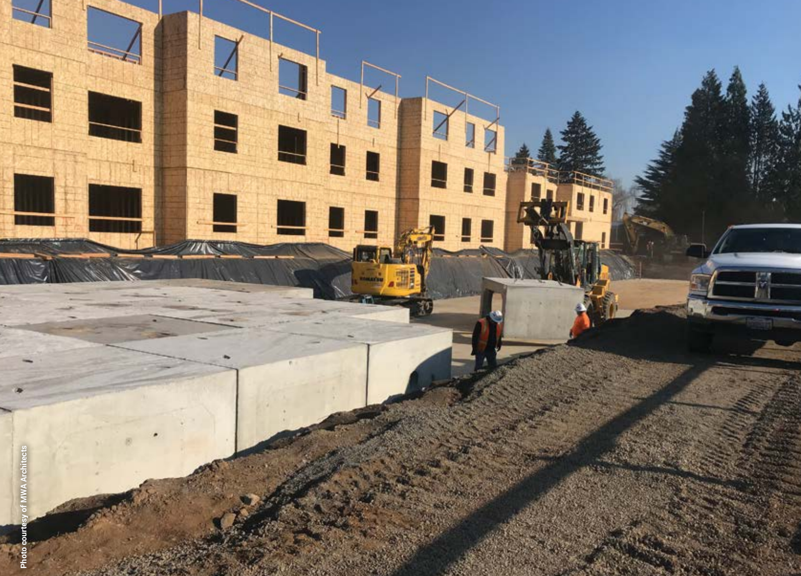
Gibbs & Olson chose a modular precast concrete stormwater detention system for a project in Vancouver, Wash. Precast overcame the site's challenges and stringent stormwater requirements.
